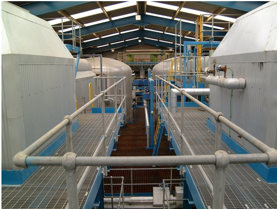
PDM fluidised bed combustion plant
